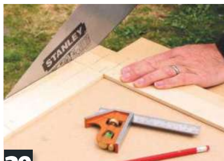
29 When glue has dried cut off horns with handsaw, leaving slightly proud. Trim flush with plane
